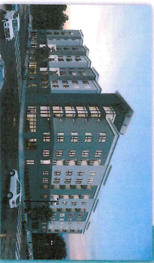
21 Washington - Carteret NJ 153 Unit Apartment & 6,500SF Retail Construction Underway Anticipated Finish Summer 2025
